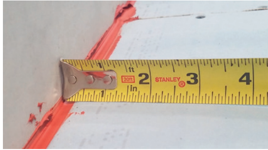
Fig. 31: Inadequate width of the sealant/gap
