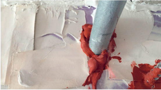
Fig. 16: Sealant not properly tooled leaving gaps in the installation
