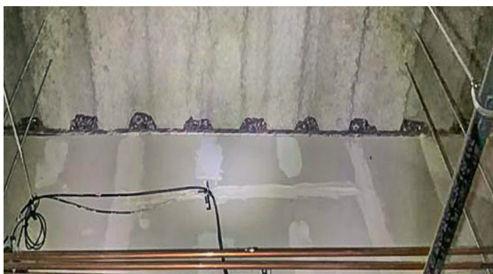
Fig. 27: Hilti CFS-TTS MD installed correctly per EJ
