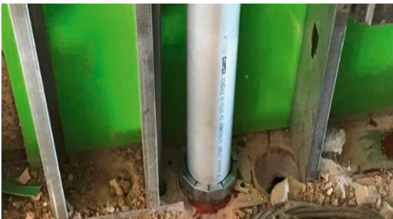
Fig. 21: Incorrect installation of collar installed on top side of floor
