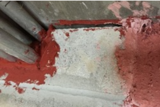
Fig. 36: Cracked sealant coating
