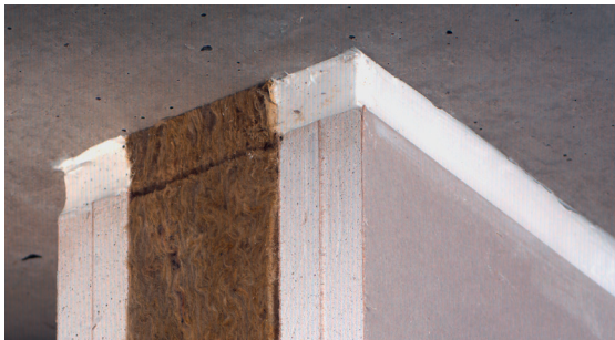
Fig. 23: Flexible fire protection sealant (Hilti CP606 - white) applied to both sides of the wall with mineral wool backing material
