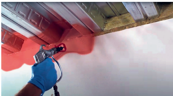
Fig. 29: Hilti CFS-TTS MD installed correctly per EJ
